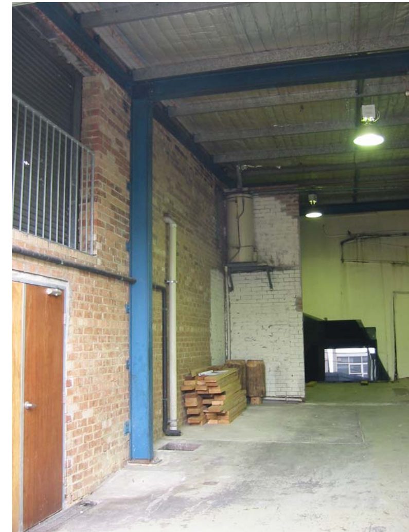
Elevated hot water tank and downpipe from neighbouring site
